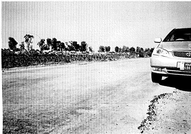
Photograph- 20 A relatively good section of old highway however broken edge requires immediate repairs
