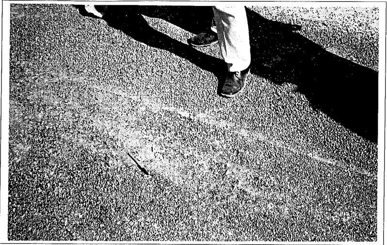
Photograph - 21 Repair work in progress but still proper bonding & embedment is not achieved
