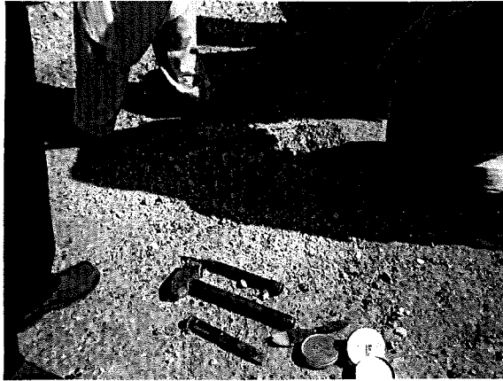
Photograph - 19 Collection of Sample to determine Moisture content of Water Bound Macadam layer
